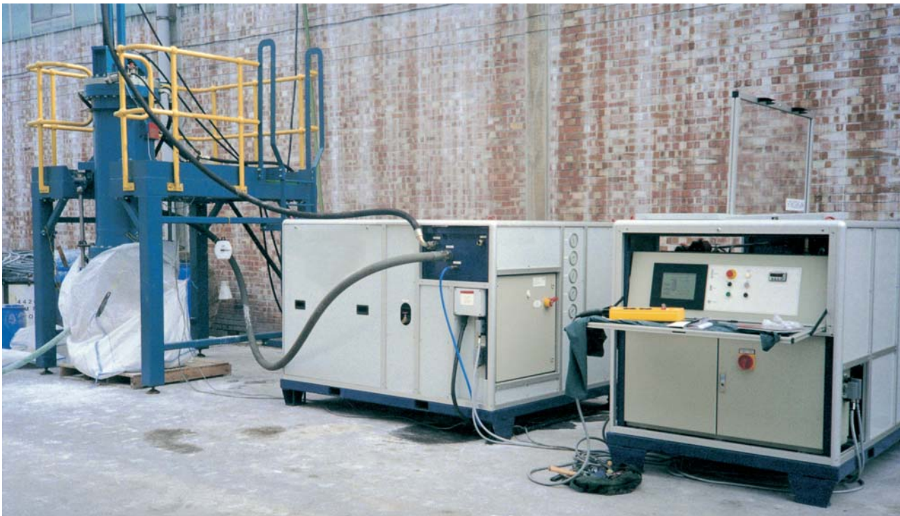
Mobile Plant Unit
