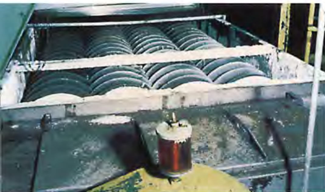
Holo-Flite® processor is used to cool sodium tripolyphosphate in a chemical plant.
