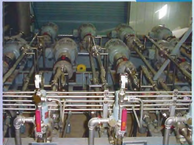
Gas Cooling De-ionized Water
