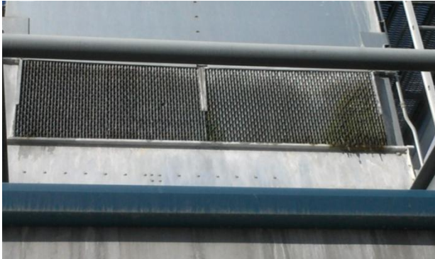
Installation date of P120 device - Scale accumulation and bio growth is evident.
