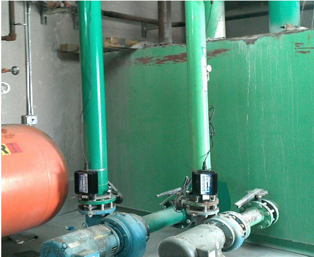
HydroFLOW P120 and P100 devices installed at the discharge from sump tank
