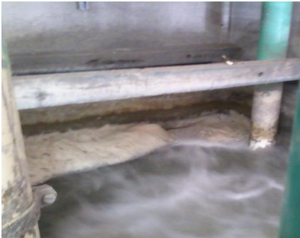
Scum, bio growth and corrosion are evident.
