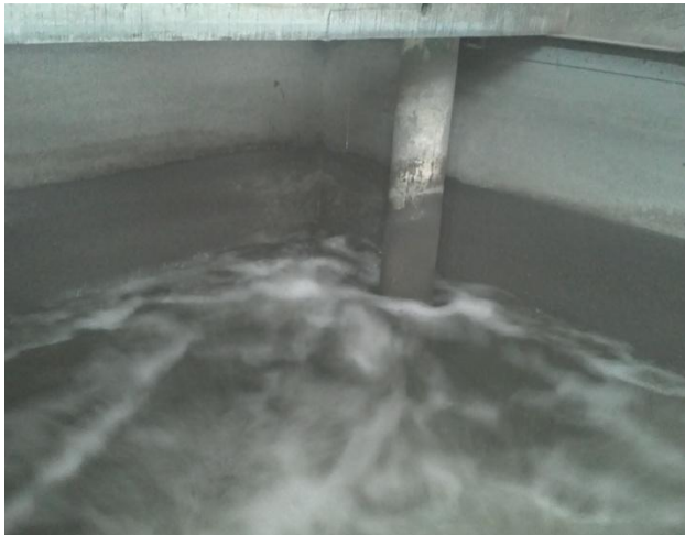
Scum, bio growth and corrosion are no longer an issue. A protective layer of magnetite has formed in place of the corrosion.
